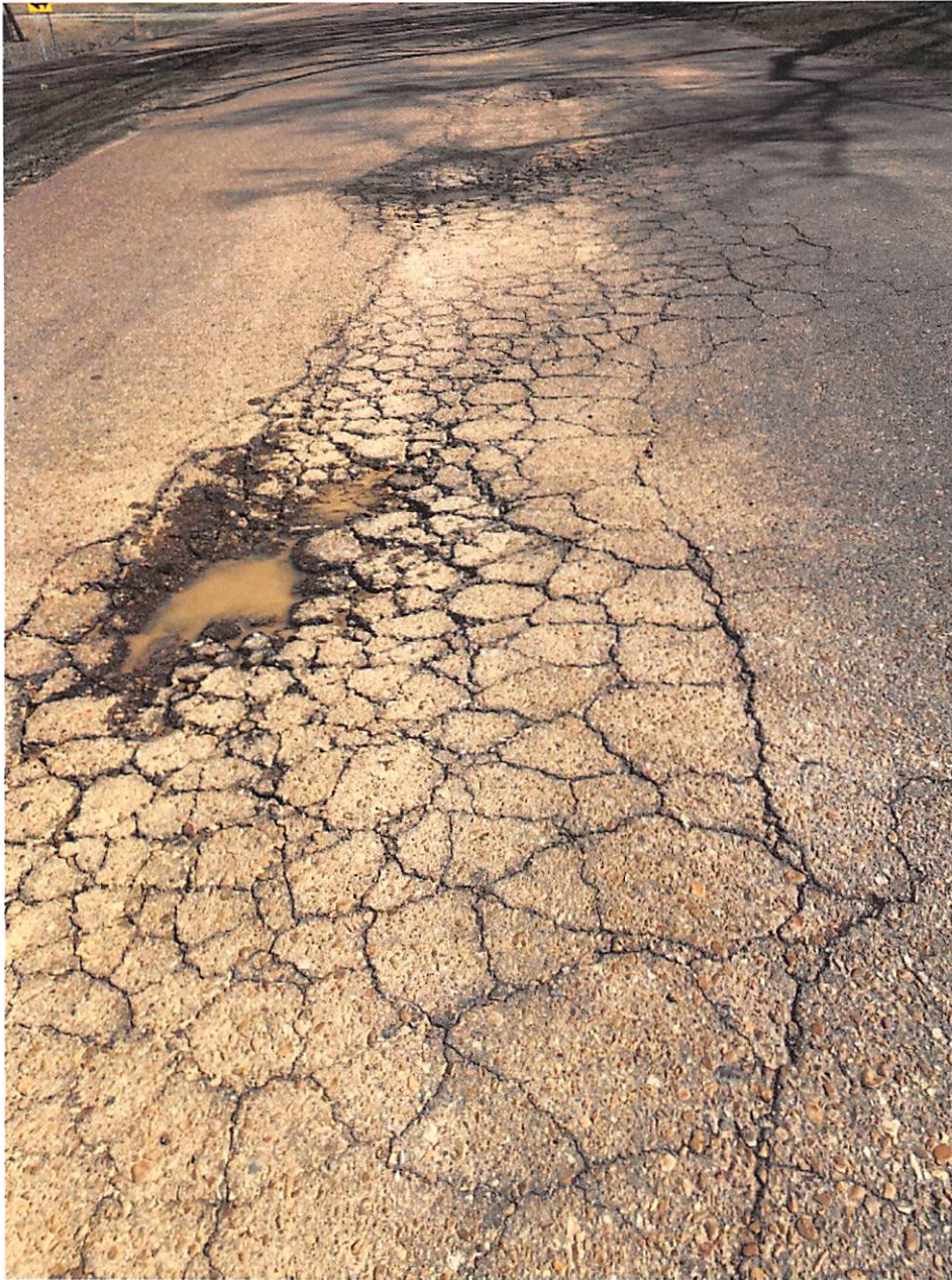
Above: Luebirdia Lane pavement condition between Falls Crossing and Catlett Road.
